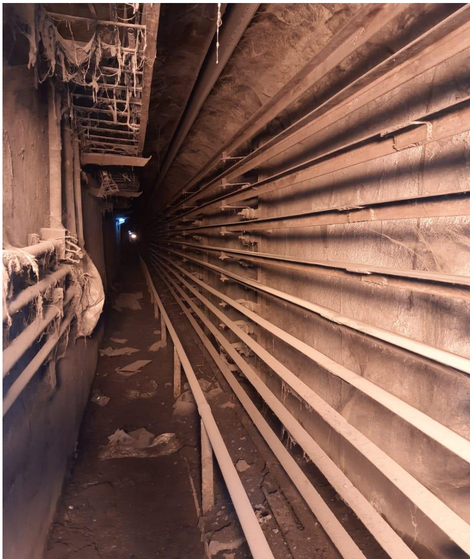
Underground bus bar arrangement for power feed to steel car and slag car
